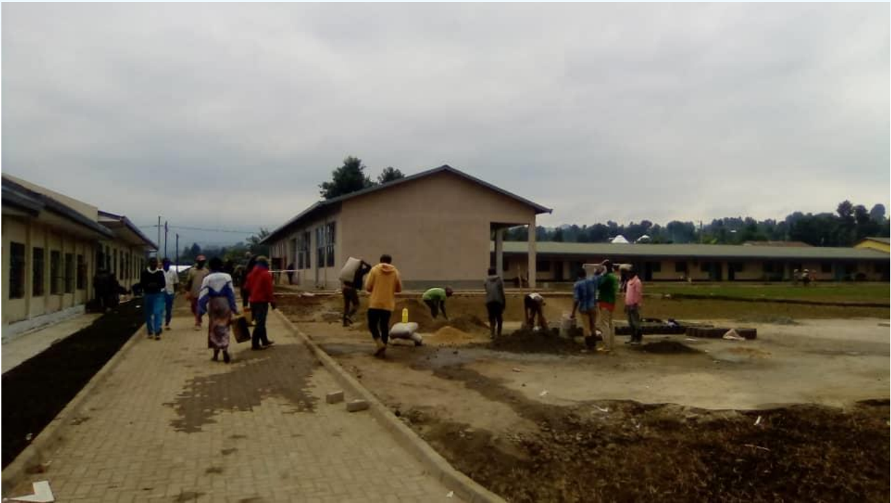
Photo NCHR, 2021: Construction works at GS Kampanga in Musanze District, Kinigi Sector
